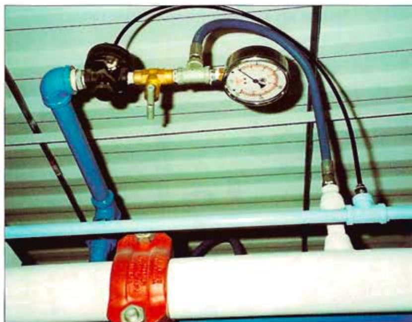
Air injector installed on conveying line
